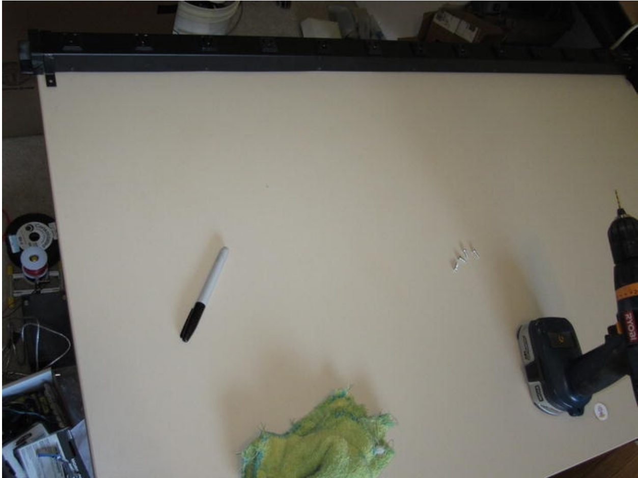
Figure 5-5. A 12-outlet power strip is attached to the back edge of the tabletop. This will provide a safe and convenient source of power for all those gadgets you'll eventually want on your bench. Tools needed for the job include a drill motor to drill out some small pilot holes for the brackets, a small drill bit, and a felt-tipped marker. Before drilling the pilot holes, align the brackets where you want them to go and use the marker to put a dot where the pilot hole should be drilled. Make sure the power strip is not plugged in when you're drilling right next to it!
